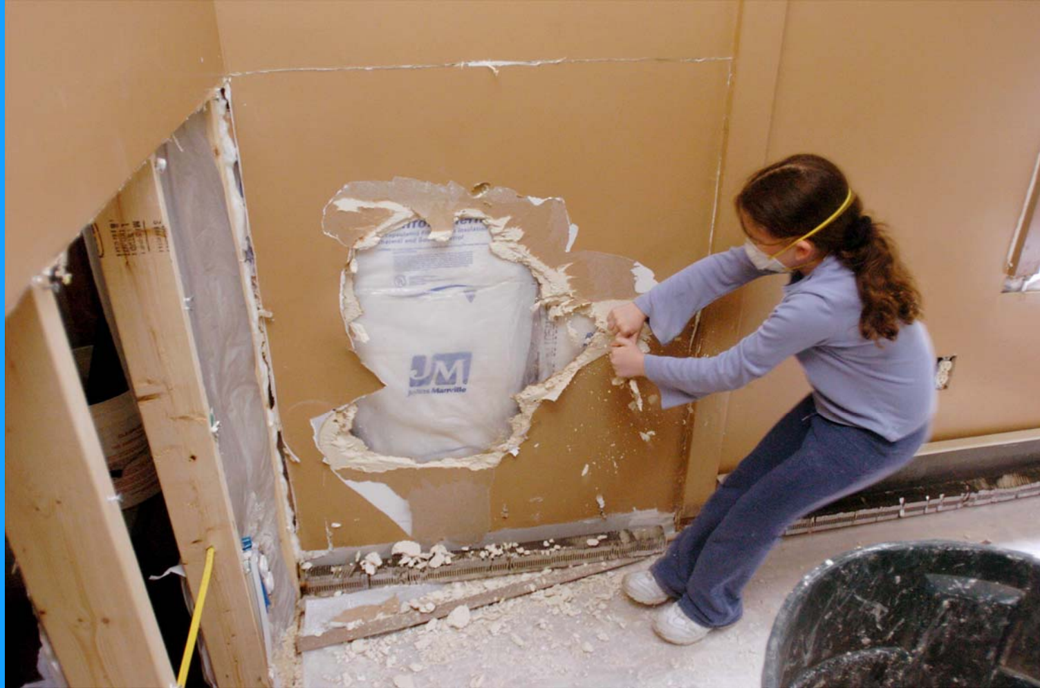
After the Flood
