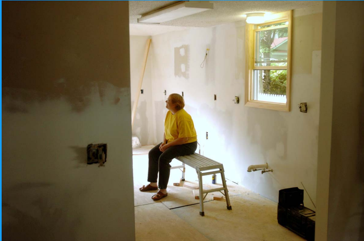
After the Flood
