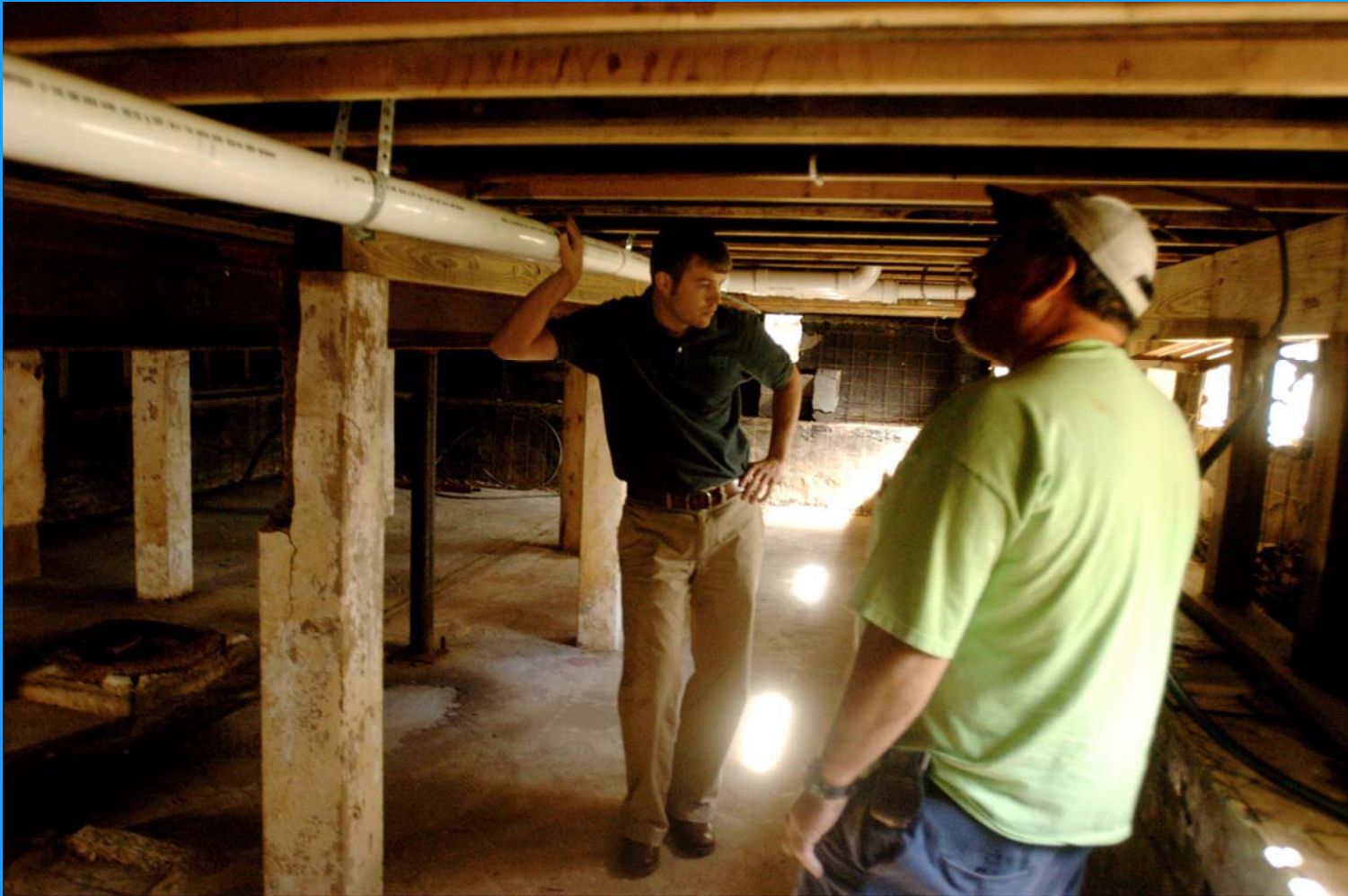
After the Flood
