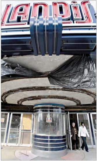
Rebuilding Landis Theater, a playhouse closed in '90, is part of the $59 million long-range redevelopment. Construction of the market could start in March for an October opening.
