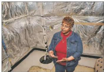
Mary Jane Plaster stands near one of the three pumps she has in her Vineland home to keep water out.
