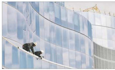
The Revel Casino under construction in Atlantic City has applied for financial help from the state.
