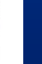
Craig Stevens (left) and Doug Anselmo of Piscataway's Department of Public Works apply hot asphalt to repair potholes on Corporate Place South on Thursday.
