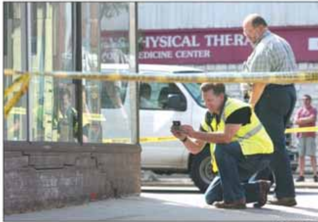
A crack at the base of the G.G. Green building in Woodbury is inspected after Tuesday's earthquake shook the area. Staff photo by Tom Heston
