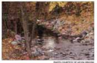
According to Kevin Origeni, this photo, from 2010, shows that the Mill Pond Dam has been in disrepair since the summer of 2010, shortly after it was repaired.
