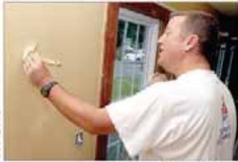
Richard's Place volunteer Fred Cohen paints a wall in the living room of Richard's Place.
