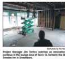
Project Manager Jim Torres watches as renovations continue in the lounge area of Tavro 13, formerly the Old Swedes Inn in Woodbury.
