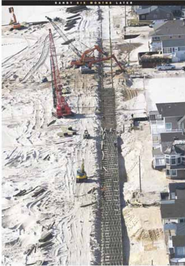
A series of heavy cranes and supports, a steel framework, takes shape in the sand in Asbury Park six months after Sandy struck on Oct. 29, 2012, as the construction resumes.
