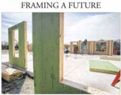
Construction work is progressing at the Trenton Housing Authority's Rush Crossing project being built at the former site of a public housing project between Lincoln Avenue and Weymouth Street.
