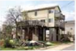
The house on Burton Avenue in Middletown is in the process of being lifted by Peter Novotny and crew.
