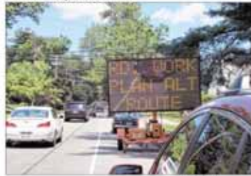
A sign on Wyoming Avenue alerts motorists to find an alternative route. Repairing work began this week on the roadway and is expected to continue through Friday, Aug. 3. Motorists will still be able to travel on portions of Wyoming Avenue because the work will be done in sections from 7 a.m. to 3 p.m. each day, but there will be detour signs and local police officers will be on site to assist with traffic control, according to the Essex County Public Information Office.
