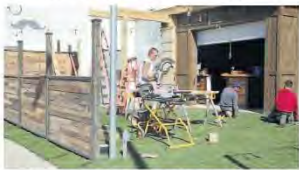
Construction continues on the Tennessee Avenue Beer Hall, expected to open later this year.
