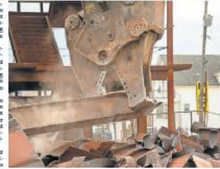
A gambler takes a photo Tuesday as crews continue the demolition of rusted steel frames in Seaside Heights. Photo by Sam DeCicco, for The Star-Ledger
