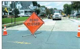
CONSTRUCTION CONTINUES: Audubon residents are starting to complain about road conditions after temporary patches begin to fail throughout town as PSE&G's gas main replacement project is ongoing.
