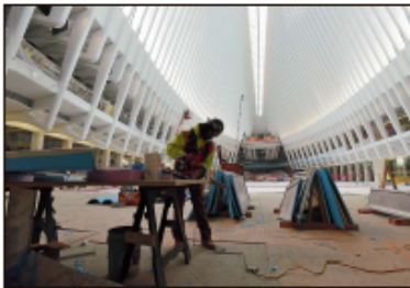
Rebuilding buses being made on the $4.6-billion World Trade Center transit hub in New York City. The Grand WTC station is expected to open in March.
