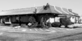
The former McDonald's restaurant in North Wildwood, which operated only seasonally, was demolished last week. Photo by Dan Wine.
