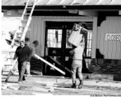
The former McDonald's restaurant at North Wildwood has been demolished and is now a vacant lot. The building was demolished last week.
